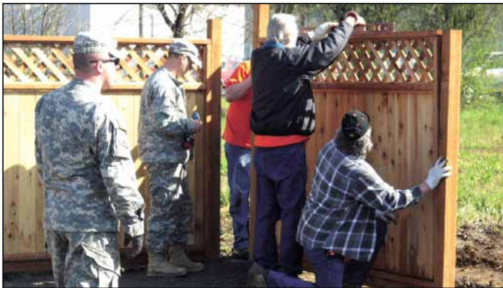
Home Depot/ Home Team, National Guardsmen and VFW post volunteers teamed up recently to construct a new fence at the Roseburg Post.
